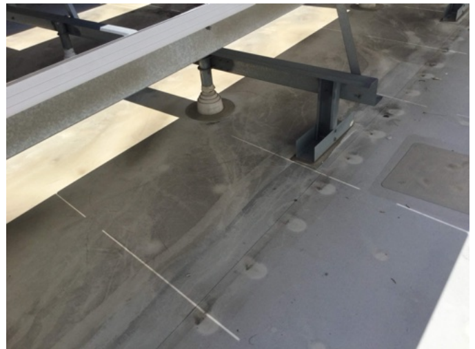
Examples of damage to a TPO roof from solar arrays.
